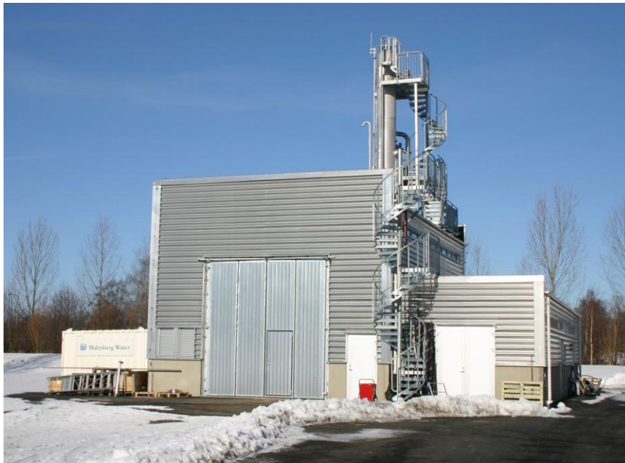
Upgrading plant GR2
